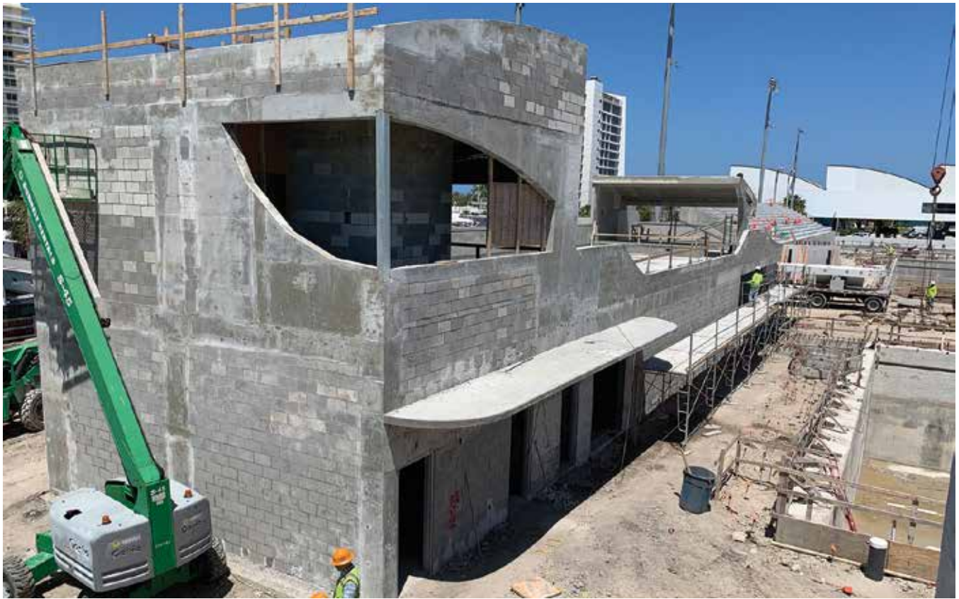
New entrance building – admissions, concessions, spectator restrooms, storage, family restroom, and 2nd floor amenity deck.
